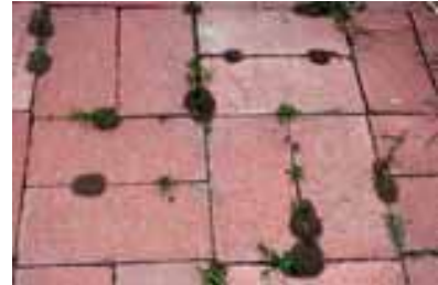
Pavement ant mounds in pavement seams
