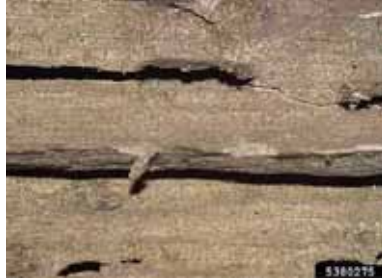
Termite damage (Gary Alpert/IPM Images)
