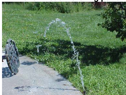
Broken head watering patio
